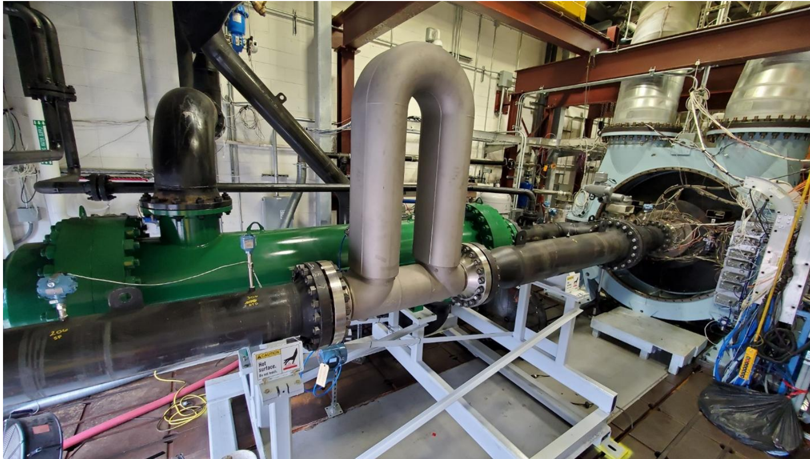
sCO 2 Compressor (Closed Loop)
