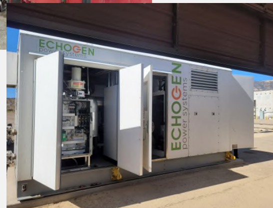
Installation at Utah San Rafael Energy Laboratory
