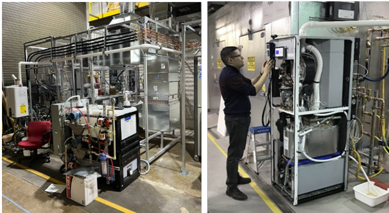
Liquid Desiccant Cooling (L) and sCO 2 -based Stirling Heat Pumps (R)
