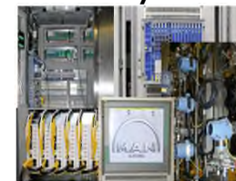
instrumentation control system
