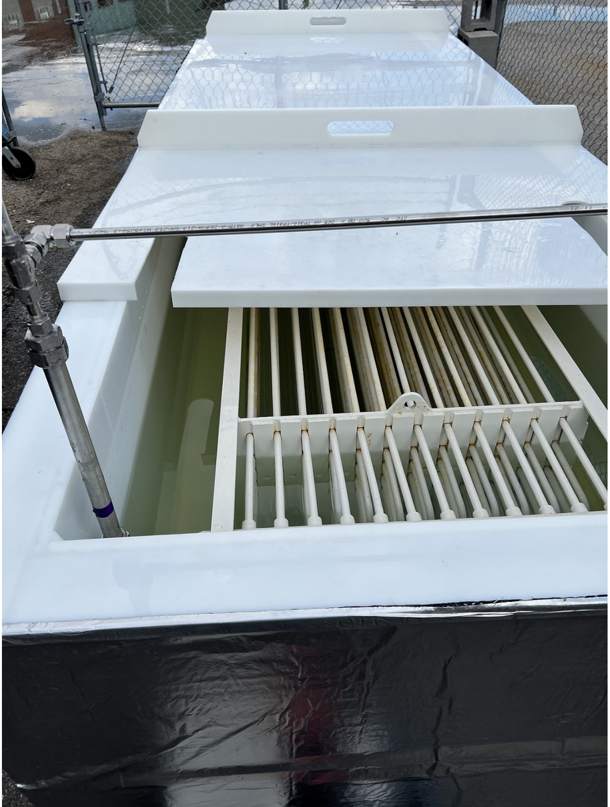
Figure 4: Installed coil and tank at Echogen lab facility
