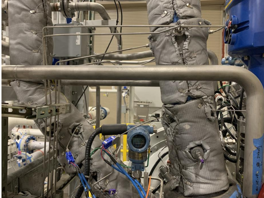
Figure 4. Suction and discharge piping instrumentation
