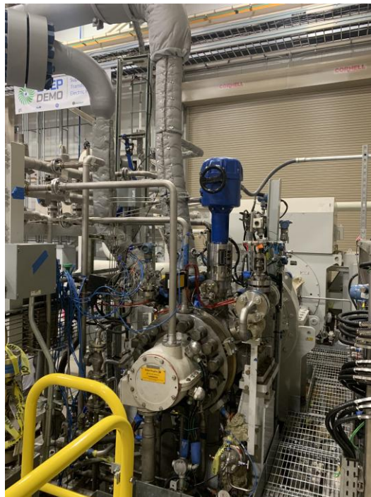
Figure 3. Main compressor with suction and discharge piping, gearbox, and motor
