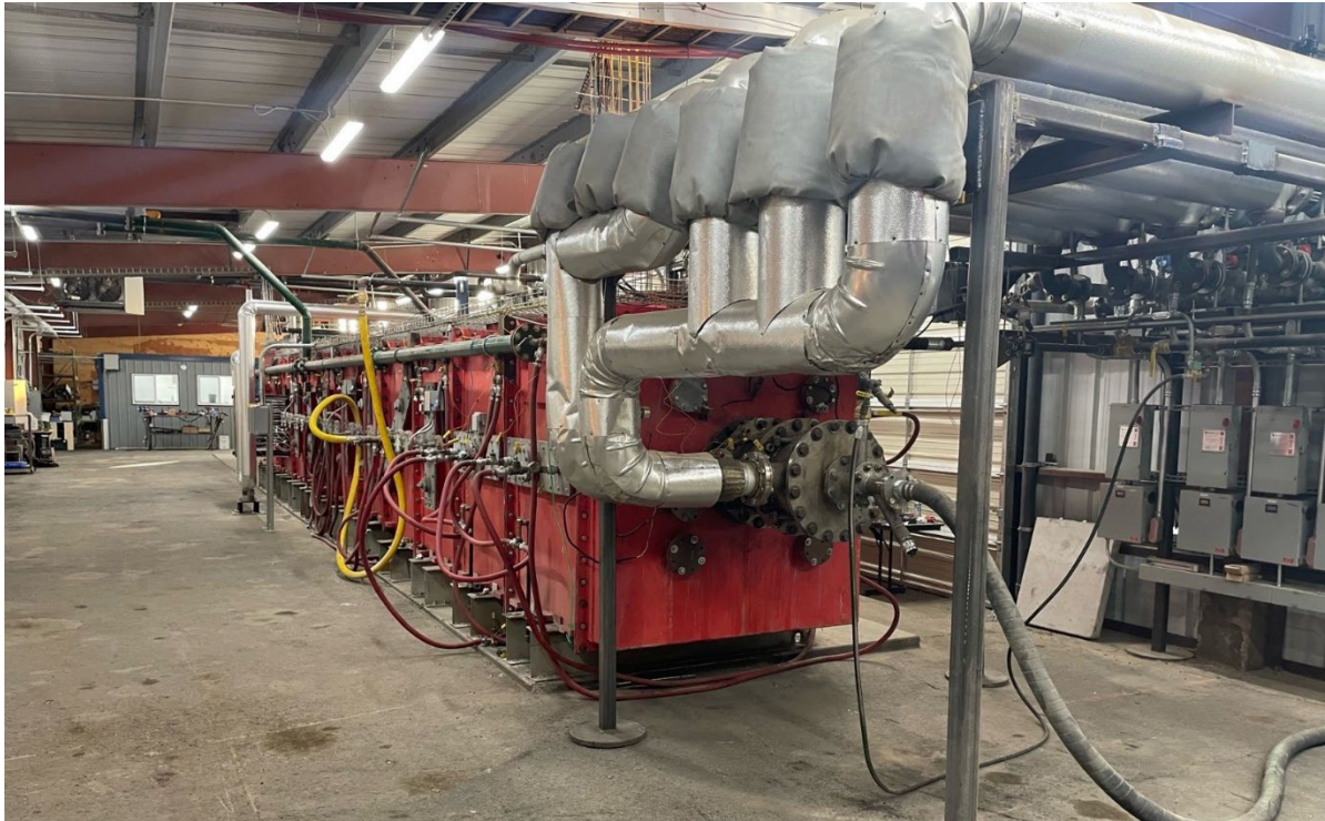
Figure 6. View of the from the front end, with burner and secondary air flow mechanisms detailed. The outlet header from the radiant section of the PHX is detailed on the far left of the furnace.
