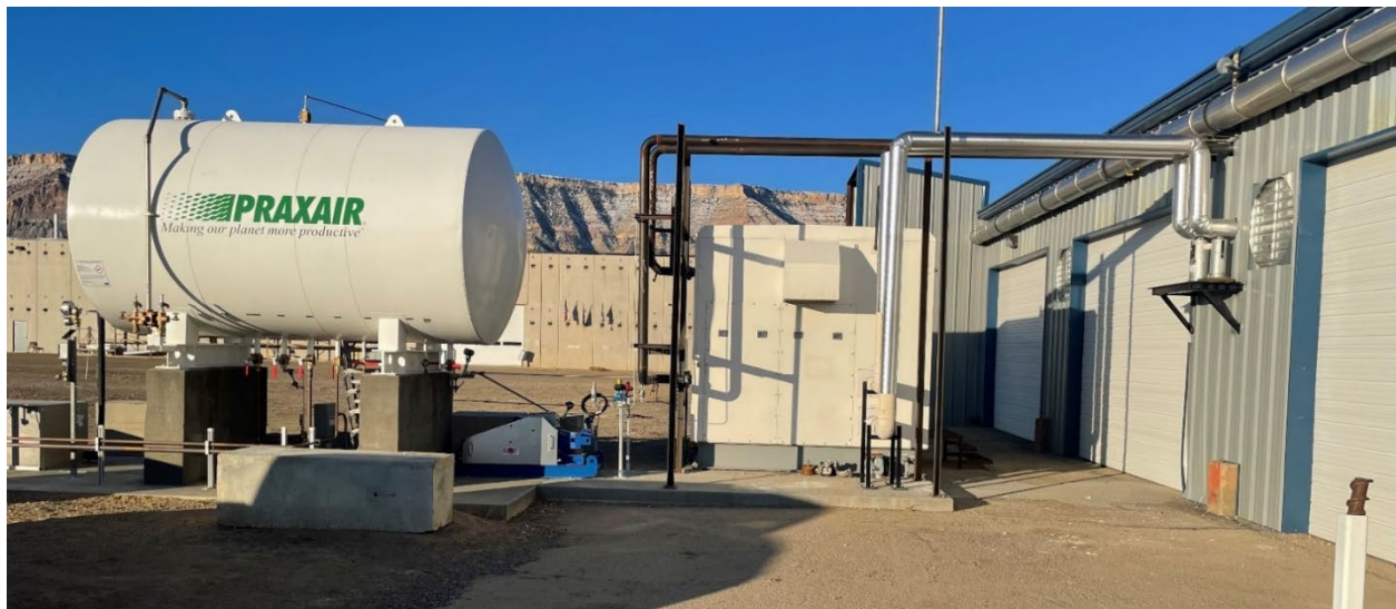
Figure 7. The thermal management system, the CO 2 supply tank and transfer pump, pictured from outside of the building.
