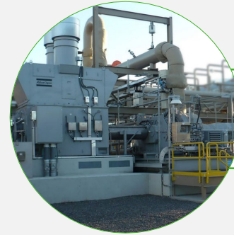
Geothermal "Stillwater", Delivery 2007
