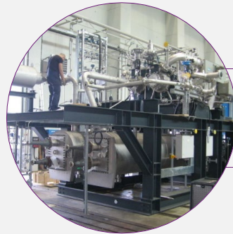
CO 2 compressor "Callide", Delivery 2008
