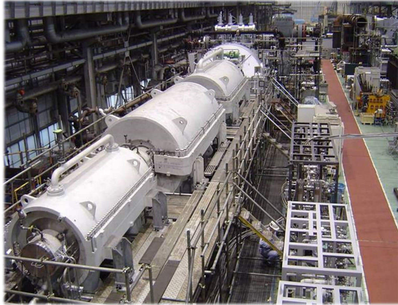
Elliott Centrifugal Compressor Train
