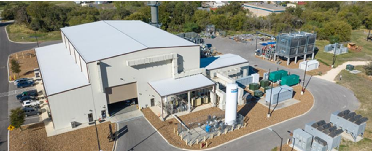
10MWe STEP facility
