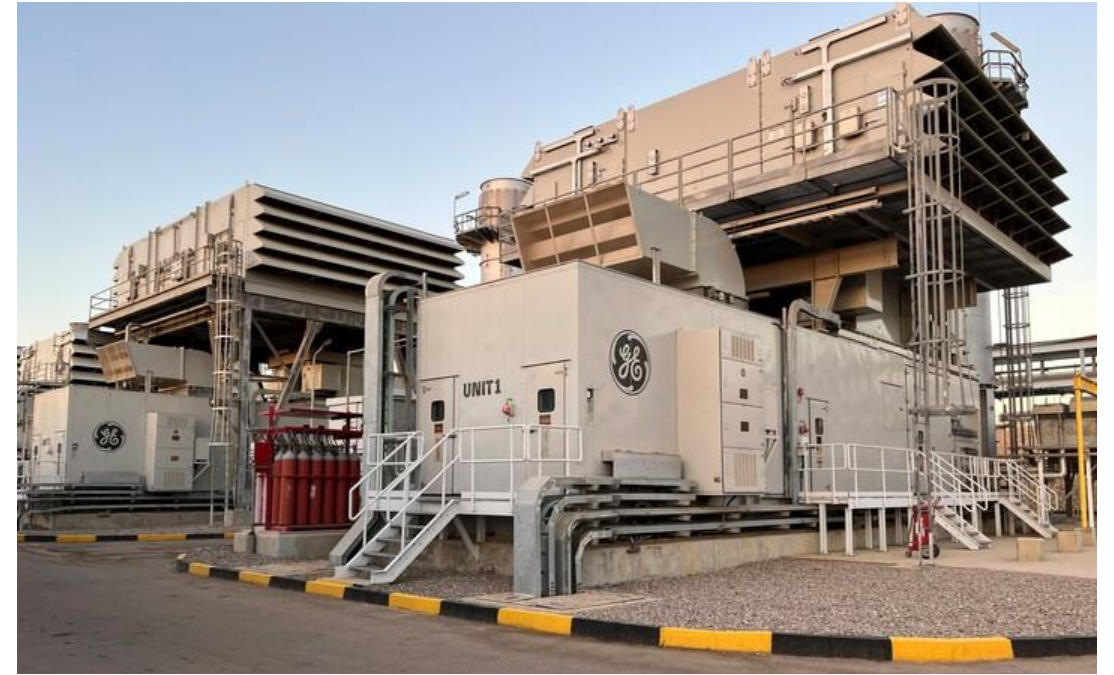
LM6000 Gas Turbine
