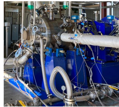
Enhanced compressor operating data
