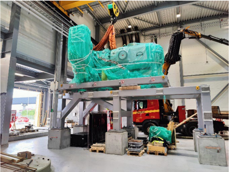
MAN Compressor @ site in Esbjerg
