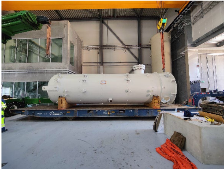
CO 2 storage tank
