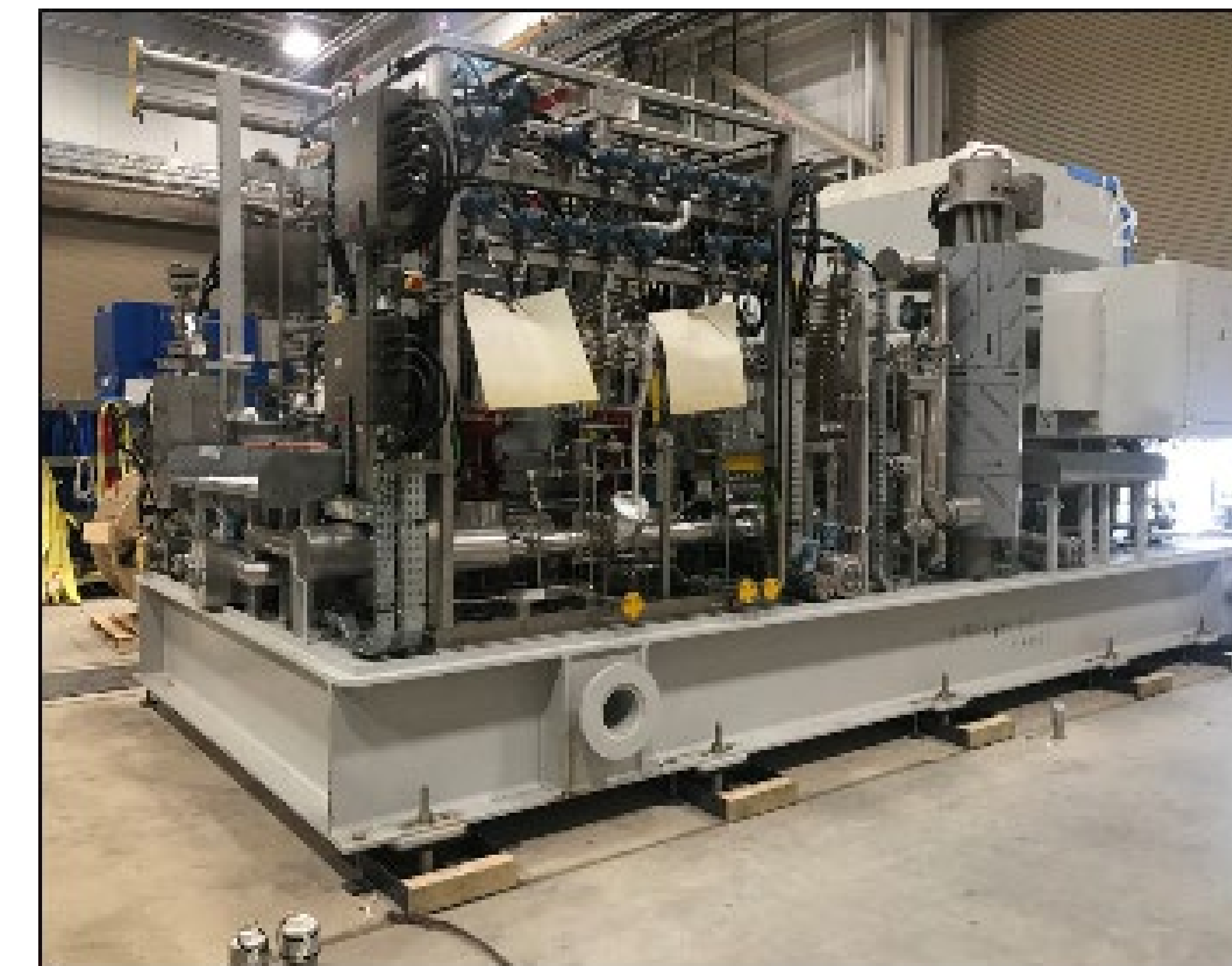
DGS installation & Warrantee work, Mar 2022
