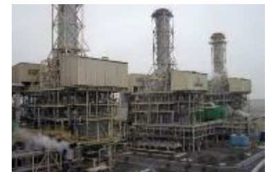
Waste Heat Recovery
