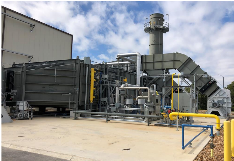
Figure 8. The 93MW th heater completed acceptance testing and is now providing heat for system commissioning.
