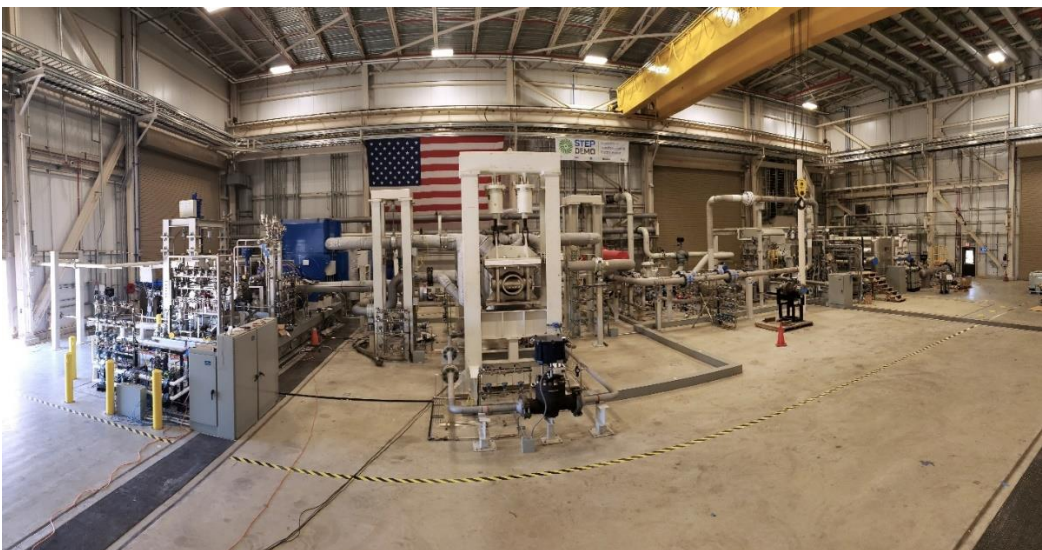
Figure 3. The STEP facility was designed with room around the equipment to facilitate component swaps and cycle reconfiguration.
