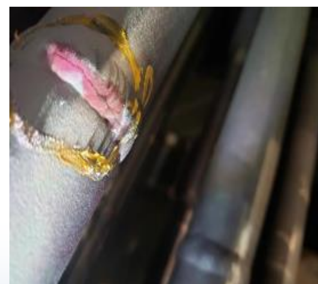
Typical Weld Crack after PWHT
