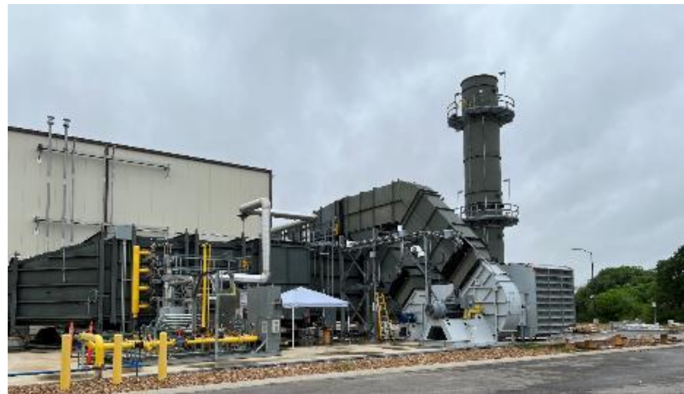
Heater at STEP Facility
