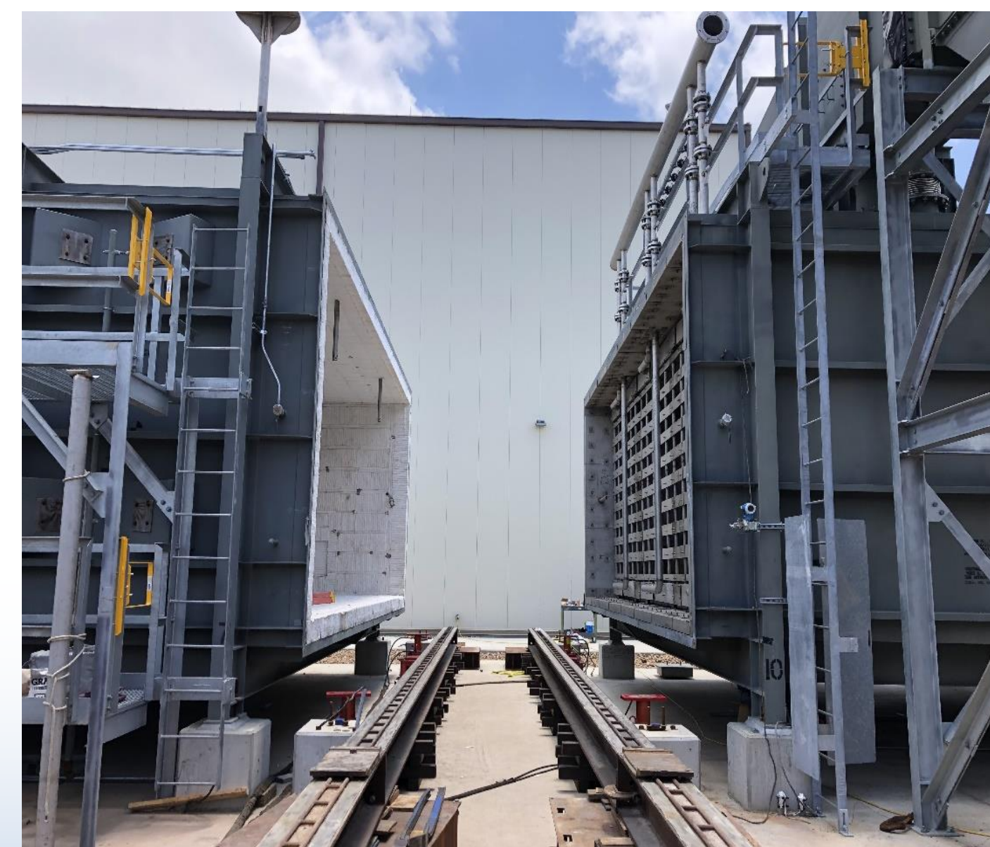
Heater Coil Installation
