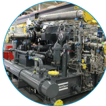
CO 2 (2 stage) Delivery 2017, demo plant
