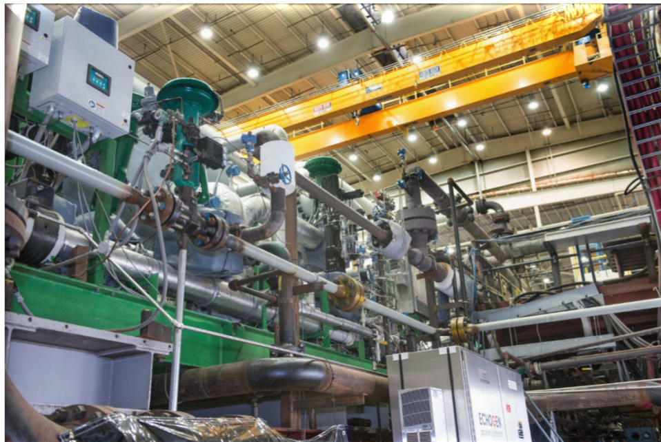
EPS100 during factory test
