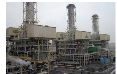
Waste Heat Recovery
