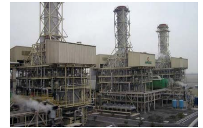
Waste Heat Recovery
