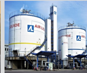
Air Liquide Liquid O 2 Storage
