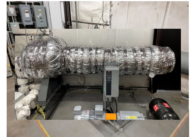
Circulating pump and recuperator in the loop
