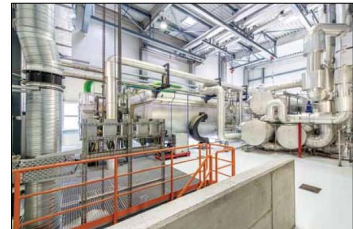
5 MWe Turboden ORC system at CRH Slovakia
