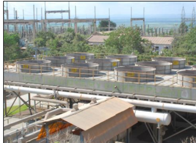
4 MWe ORMAT ORC system at Ultratech Cement, India
