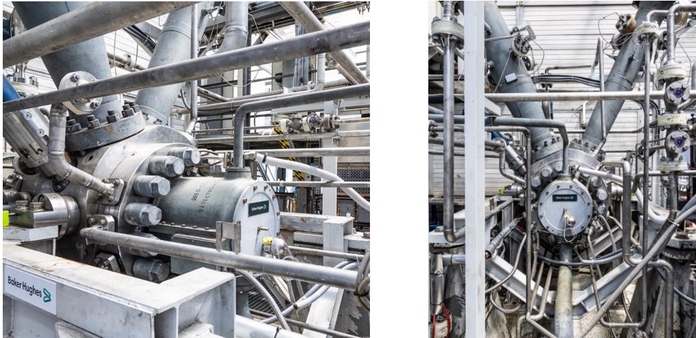
Figure 3 – Prototype installed on the test rig at the Baker Hughes facility in Florence, Italy
