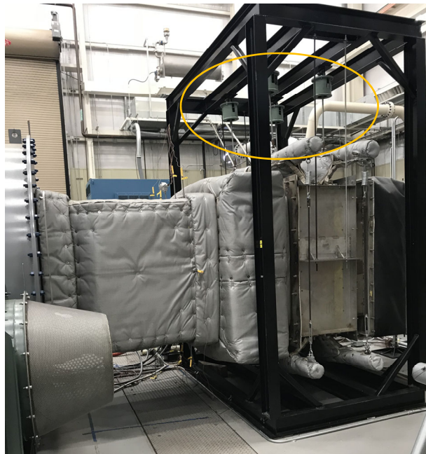
Heater supported with spring hangers
