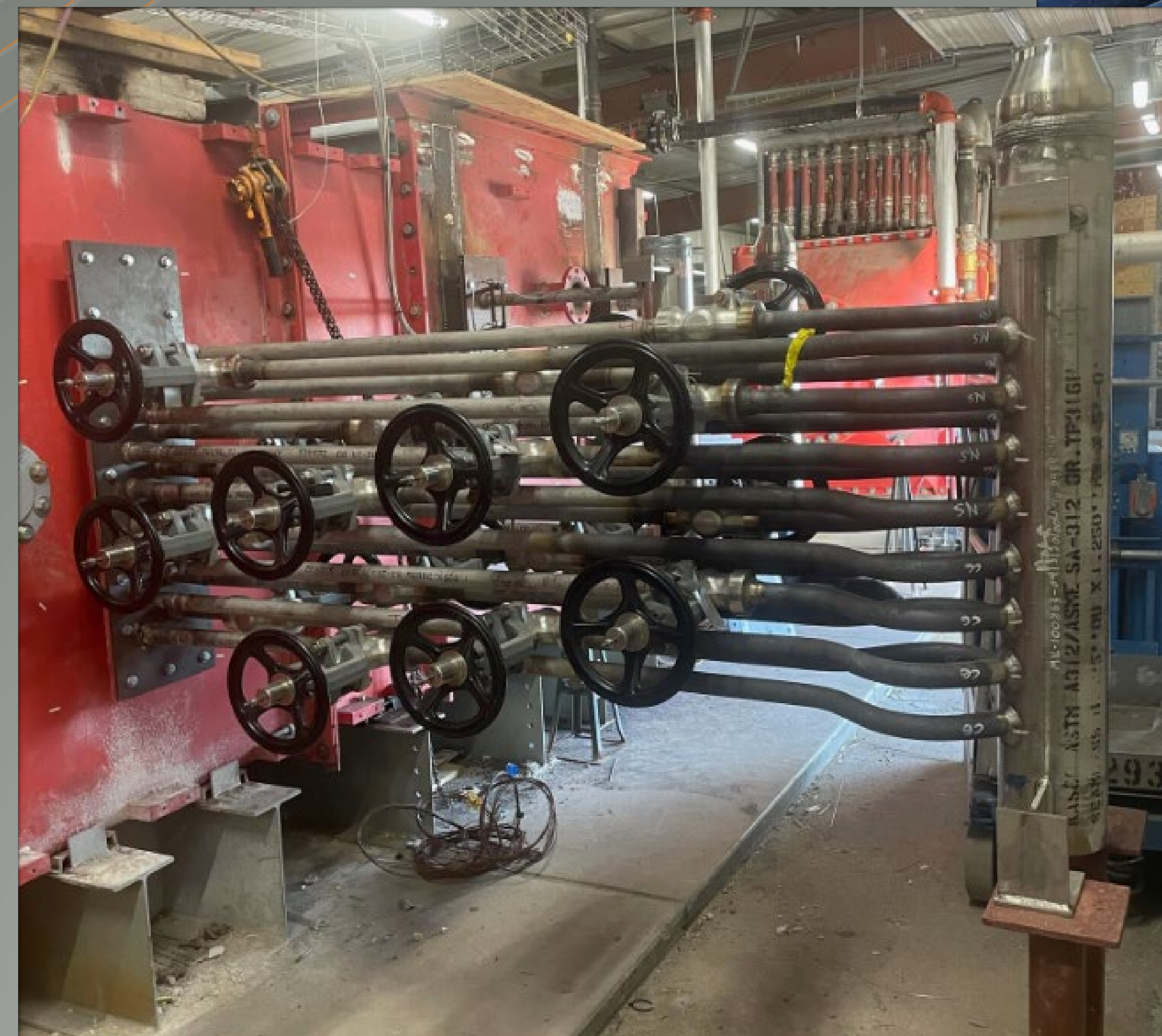
Fig14: (Right) Flow Balancing Valve Installation with Outlet Header.
