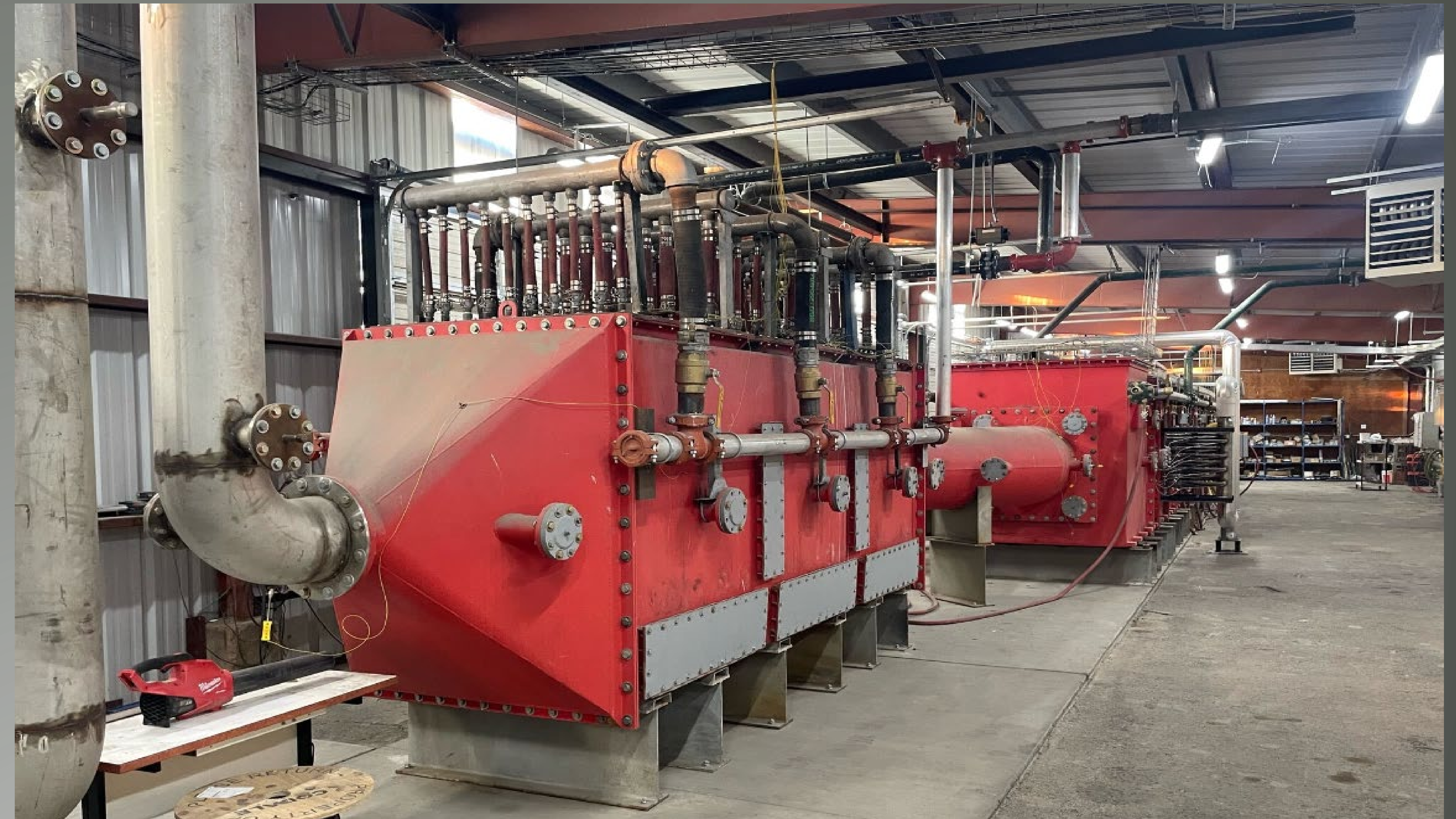
Fig3: L1500 Furnace. Convective Section (in foreground) with Exhaust Piping and Cooling Manifold.
