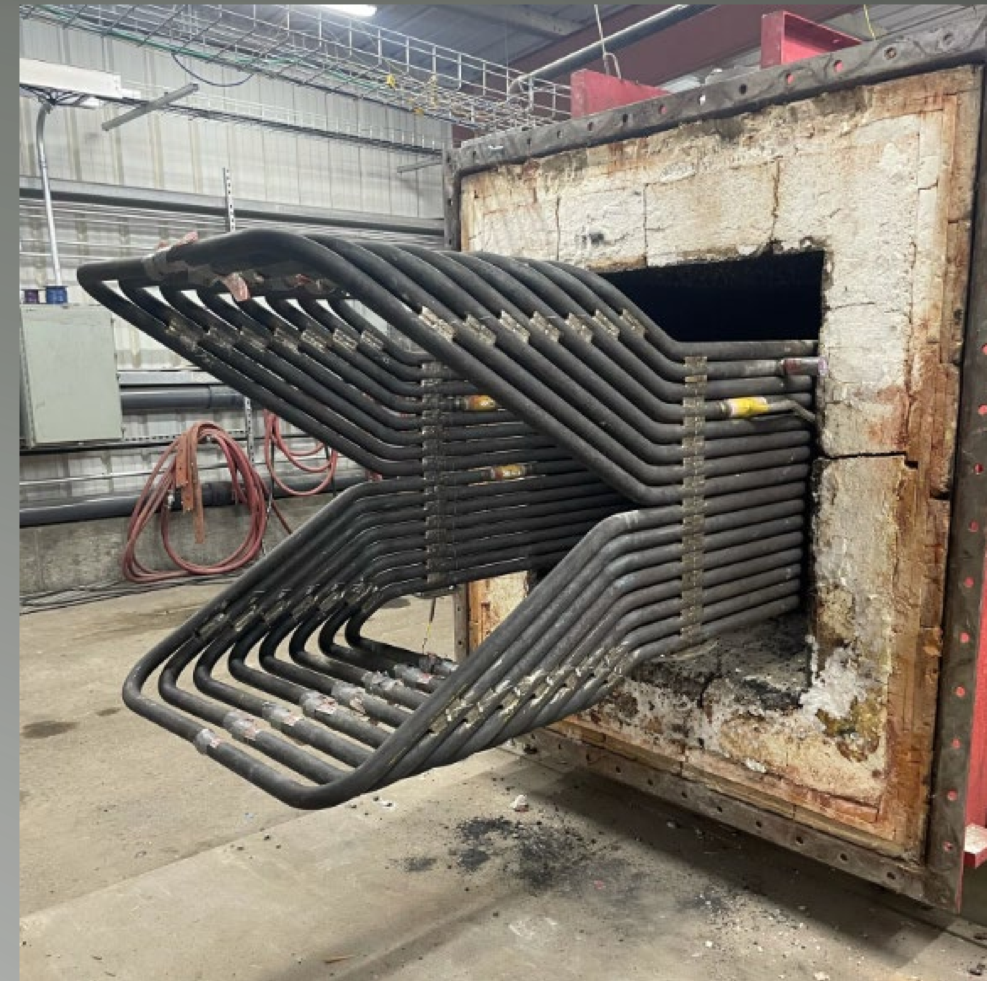
Fig11: Primary Heat Exchanger (PHX) Installation
