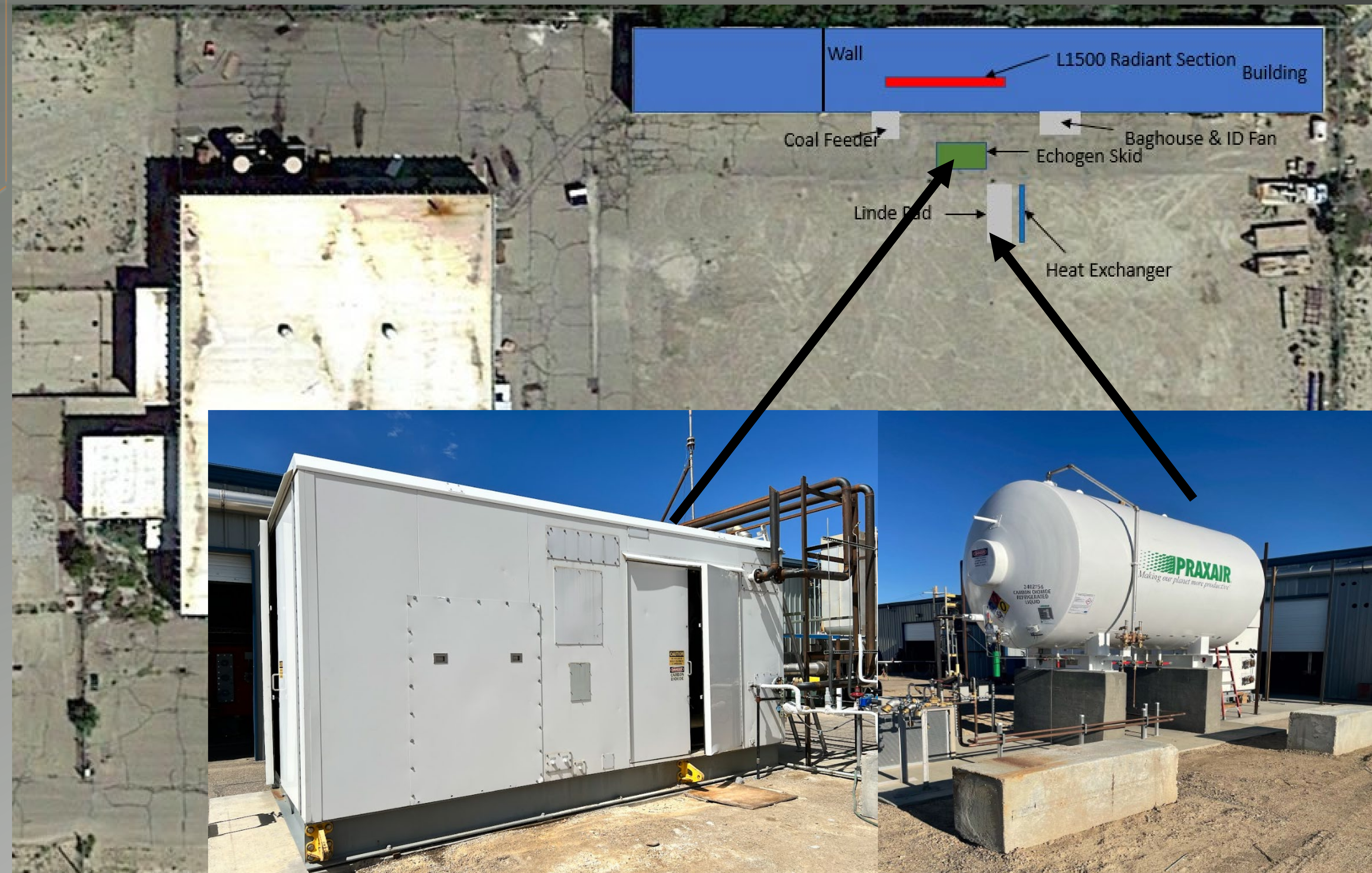
Fig5: Echogen Power Systems Thermal Management System Installed at SRERC.
