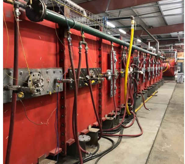
Figure 3: L1500 Radiant Section (Foreground) with Transition and Convective Sections (Background)
