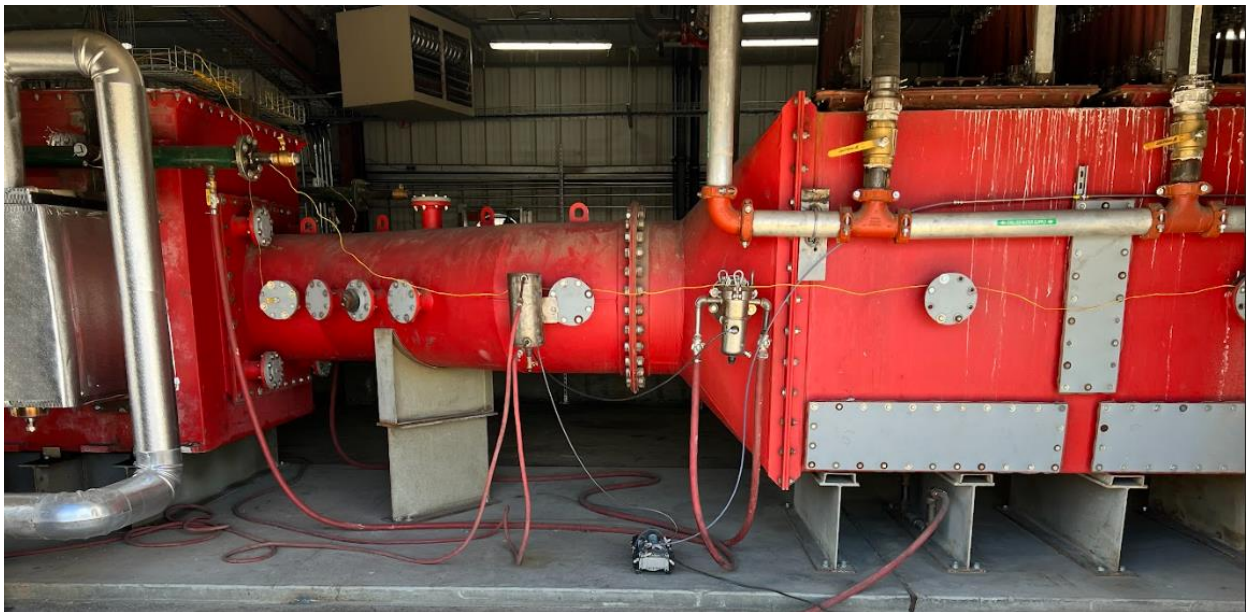
Figure 4: L1500 Transition and Convective Sections
