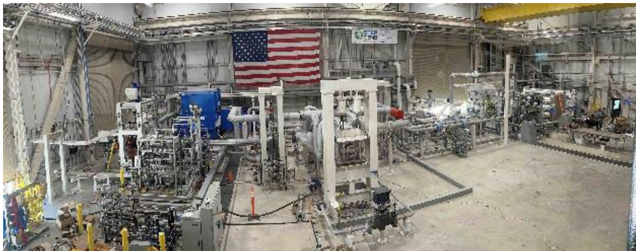
Figure 4: Power cycle equipment
