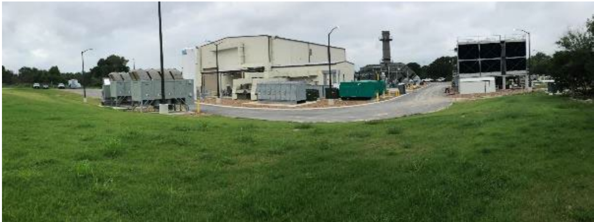
Figure 3: STEP USA facility building (middle), cooling towers (right), heater and stack (middle), load banks (left)
