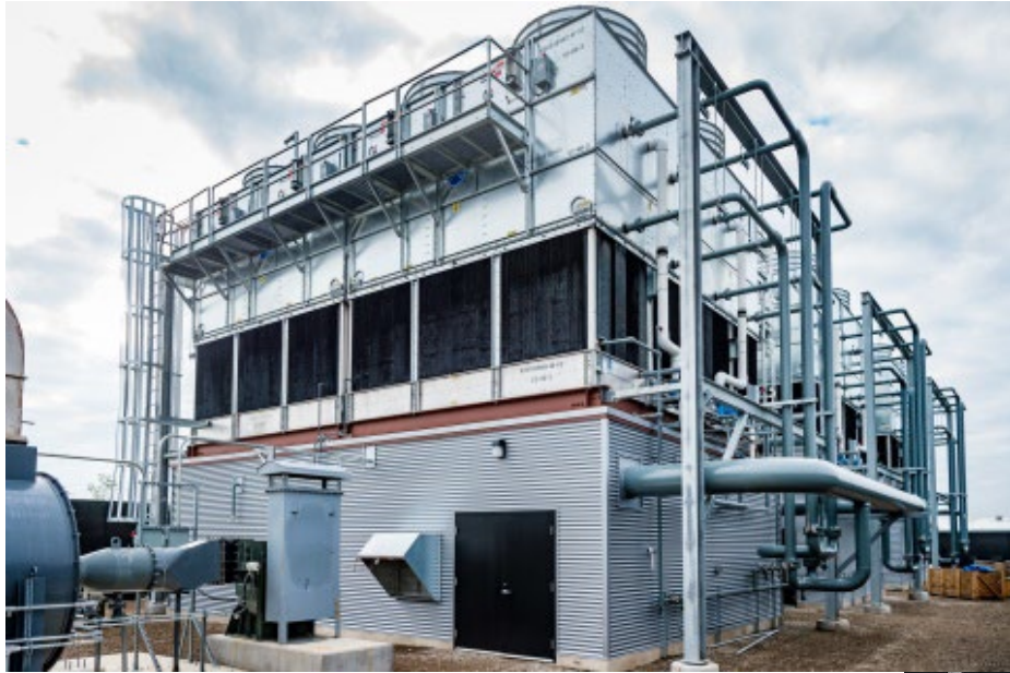
Cooling towers – 12MW
