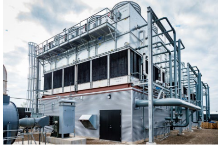
[Cooling towers – 12MW]
