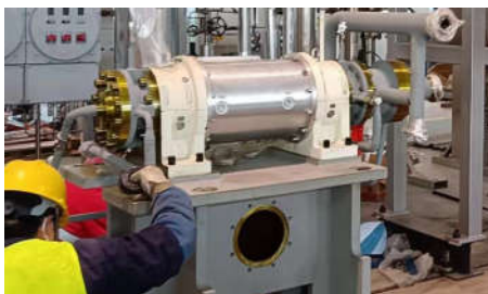
The motor and compressor
