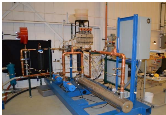
Heat Exchanger Test Loop
