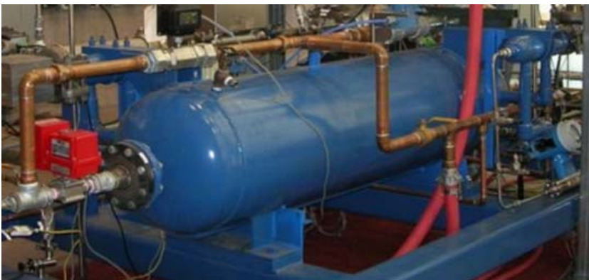
Compressor/ Seal Test Loop
