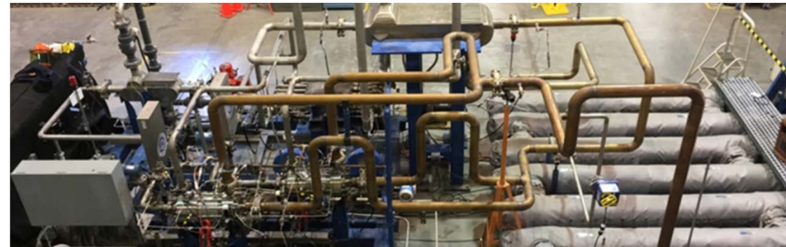
sCO 2 System at Sandia NL Illustrating Piping Complexity
