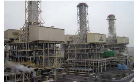
Waste Heat Recovery
