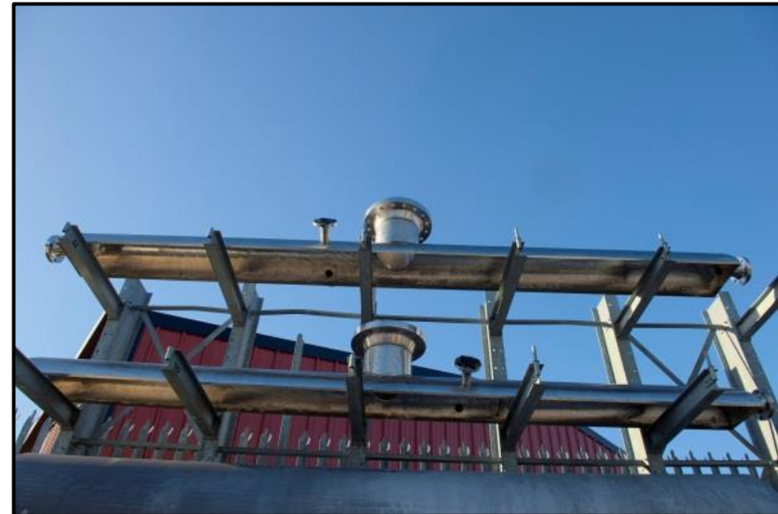
Headers, nozzles, flanges
