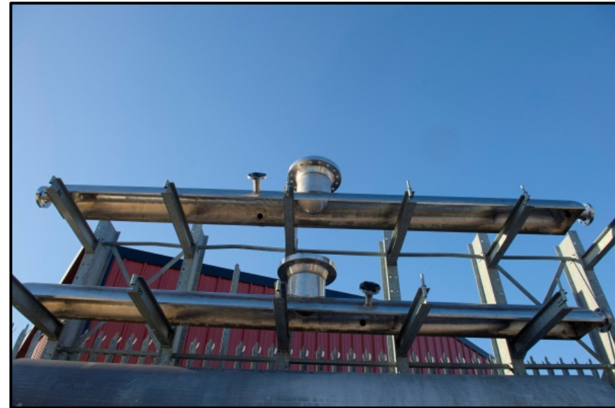
Headers, nozzles, flanges
