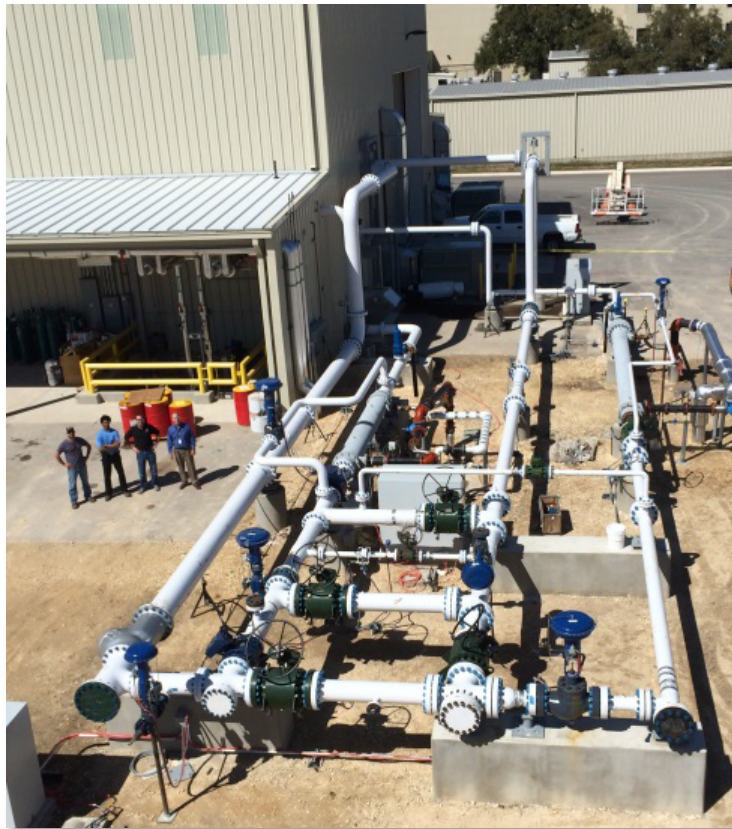
Figure 8. Existing CO 2 Pipe Loop
