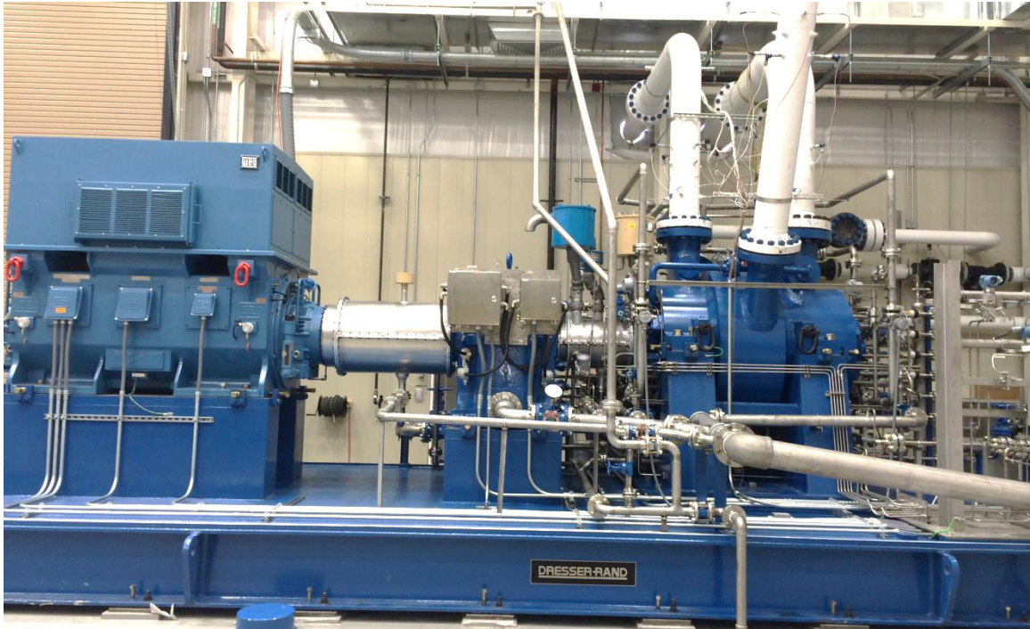
Figure 7. Exist 3 MW CO 2 Compressor
