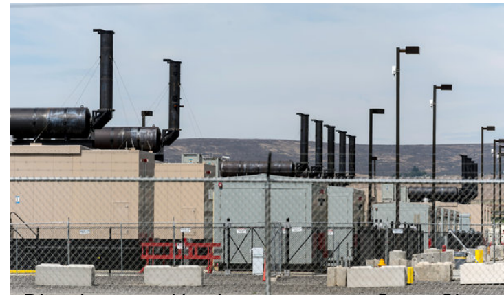
Diesel-powered backup generators, Santa Clara
