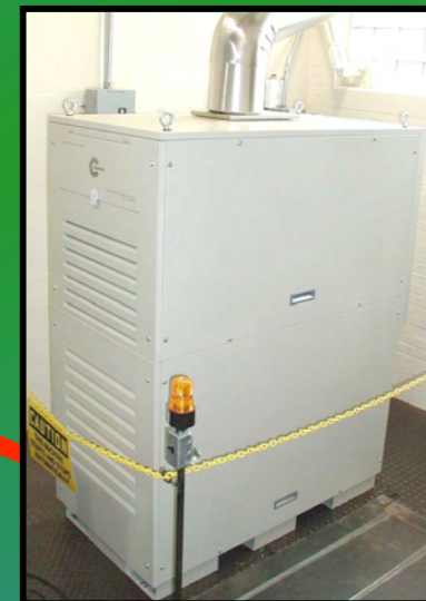
Capstone MicroTurbine proof-of-concept & environmental durability test facility
